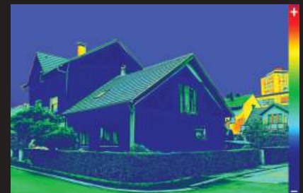
THERMAL IMAGE OF THE SAME STRUCTURE BUILT WITH 1/2" (R-3) OF CONTINUOUS INSULATION
